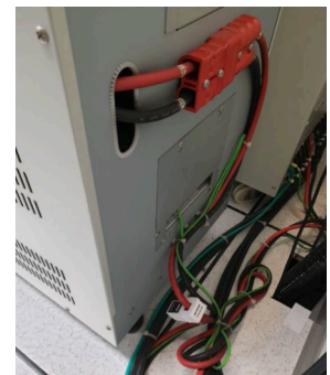
UPS Power Consumption Monitoring
